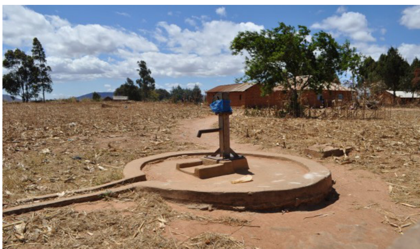
Picture 31: A Broken Water Pump at Mlanda Village
