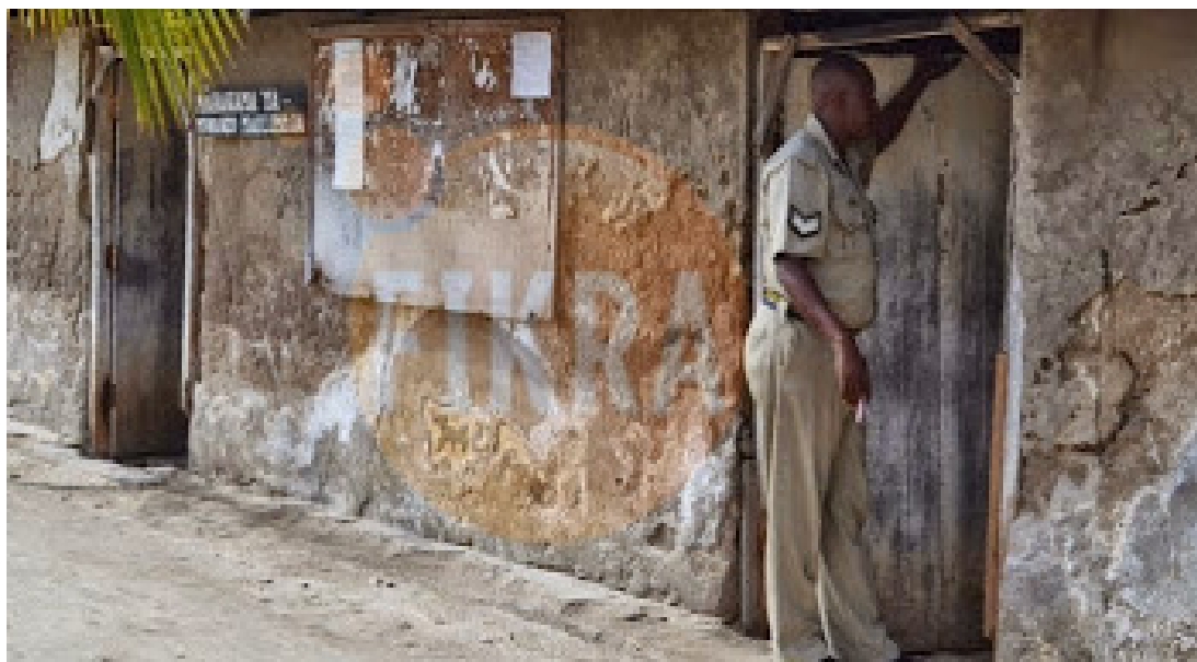
Picture 10: Dilapidated building hosting the Kibaha Primary Court
