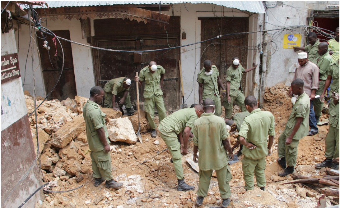
Picture 89: Kikosi Cha Zimamoto were in pursuit of removing the rubble to see if anyone was under the rubble following the collapse of a three-storey building at Jaws Conner, in the Stone Town on 19th November, 2014.
