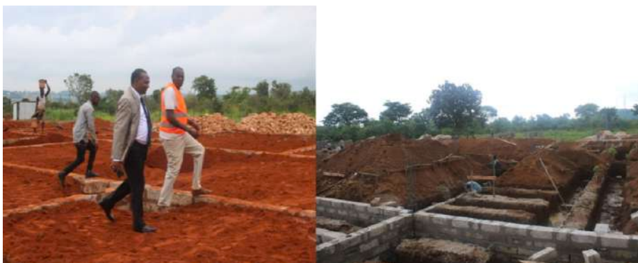
Picture 6: Principal Judge of the High Court of Tanzania – Kigoma Zone, Judge Lameck Mlacha (in suit) inspecting ongoing construction of court buildings in Kigoma
