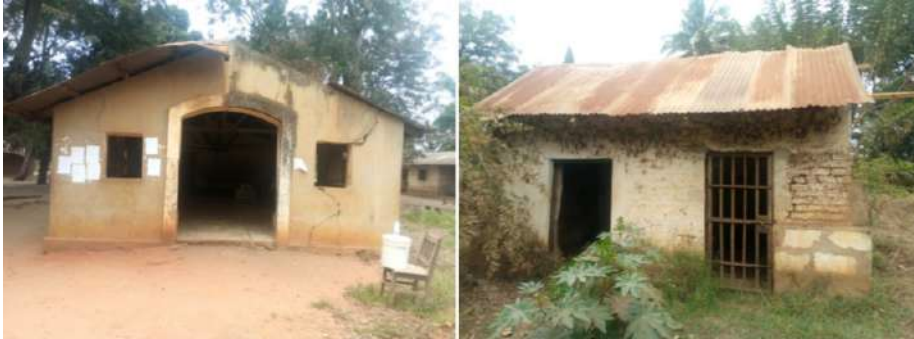
Picture 32: Right: Rudewa Primary Court building found in dilapidated condition; Right: An unused lock-up cell at the court, also in dilapidated condition
