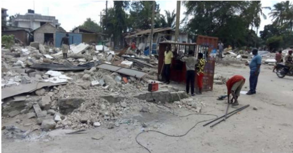
Picture 25: Demolition in Kimara Area in Dar es Salaam (Picture by the IPP Media)
