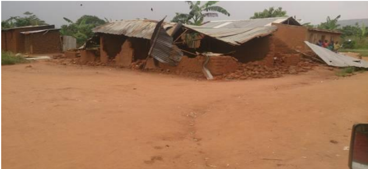
Picture 26: The demolished house of the CCM Candidate one Abdallah Rugamalira who was declared the winner of the Village Chairperson post on the 17 th December 2014 local government re-election.
