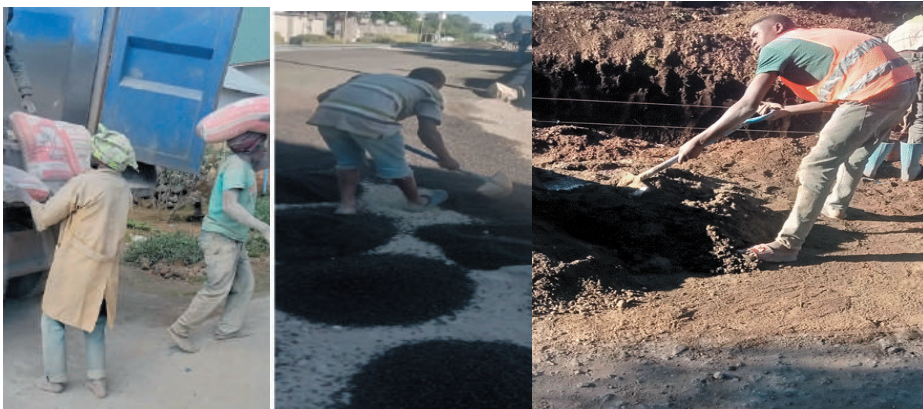
Picture 3.16: Casual workers observed working without PPE in Mbeya
