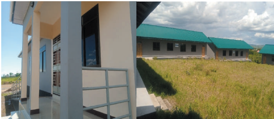
Picture 6.4: A teacher house (right) constructed in Nyamongo Tarime DC (left) and an ongoing construction of a classroom in the district(right), both supported by North Mara Gold Mining Limited
