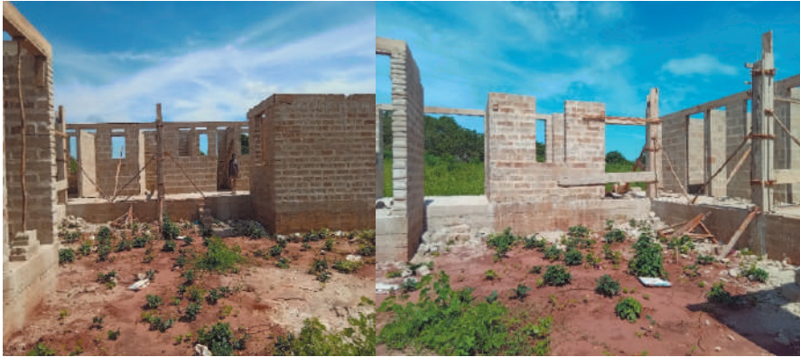
Picture 6.9: Ongoing construction of a dispensary in Hiari Village, funded by Dangote Cement PLC
