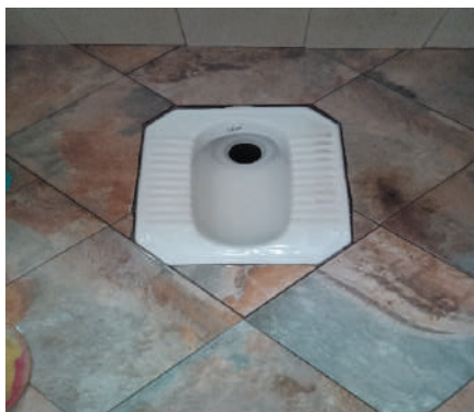
Picture 3.5: A toilet without a flushing system observed at Petro Africa in Masasi TC, Mtwara
