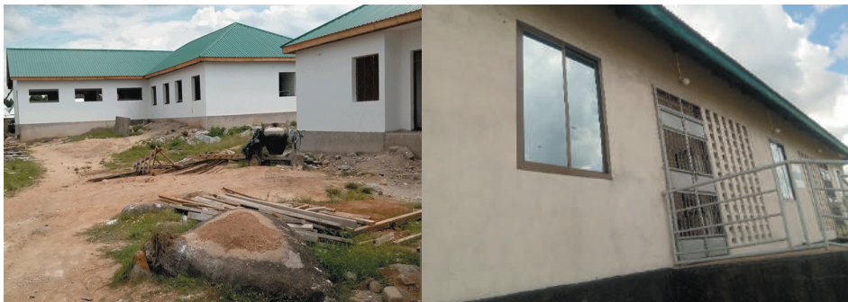
Picture 6.7: Ongoing construction of Nkome Health Centre (left) in Nkome Ward, Geita DC, supported by GGML and a dispensary in Nyamongo, Tarime DC (left) constructed with the support of North Mara Gold Mine Ltd
