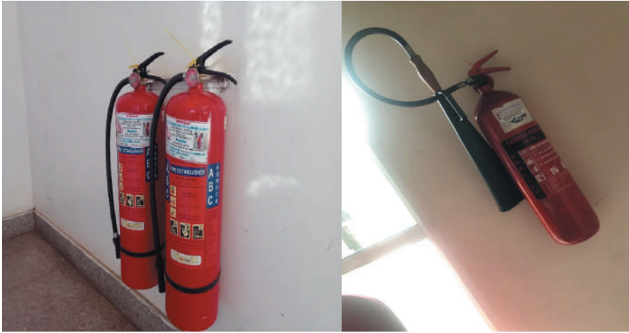
Picture 3.8: Fire extinguishers observed at Dangote Cement PLC in Mtwara (left) and Flomi Hotel in Morogoro (right)
