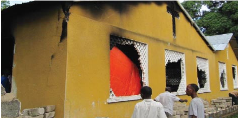
Tanzania Assemblies of God (TAG) church at Kariakoo in Unguja Urban District which was partly damaged after unknown arsonists set it on fire during the political riots occurred between 26 th May and 28 th May, 2012.
